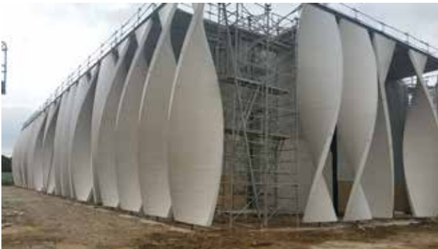
Precast concrete facade of multi-sports hall building for a polytechnique school in France.
