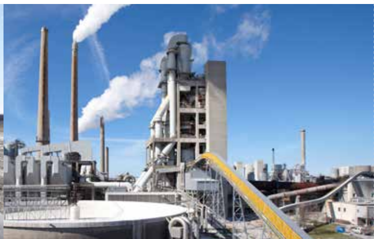
Kiln 87 - cyclone tower
